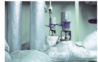
Air conditioning system
