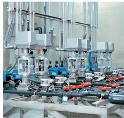
PSN installed in a water treatment plant
